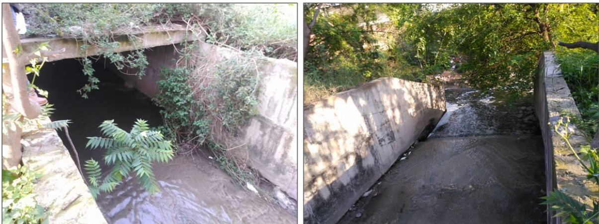
Figure-7 Discharge of sewage of Manimajra into MDC drain.
