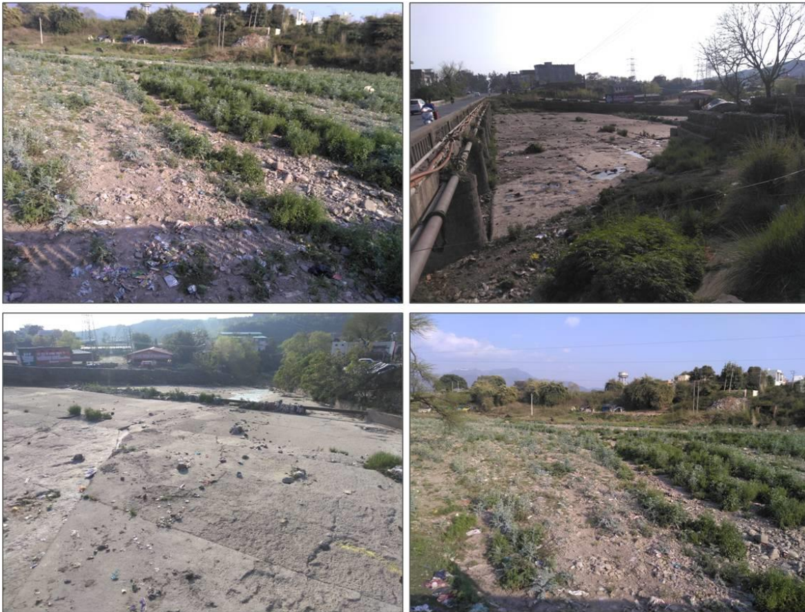
Fig 5:-The latter plastic, packaging material, clothes etc. seen lettered in river bed and mushrooming of Jhuggis.
