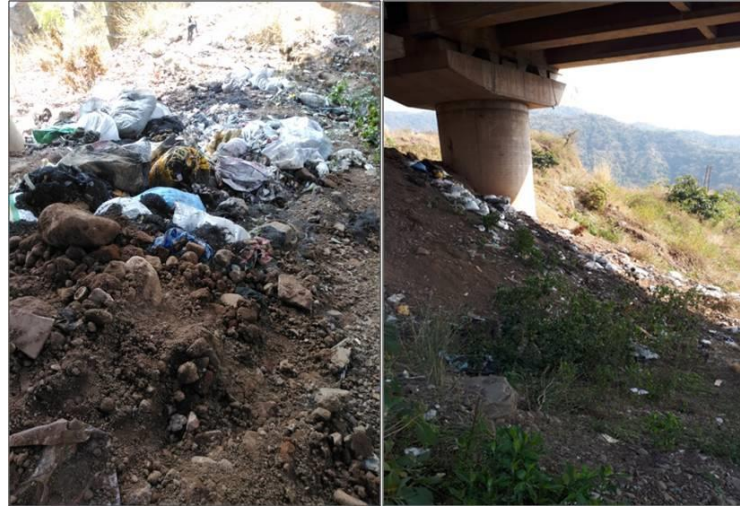
Figure-2 used bags thrown on bank of sub-drain under bridge of Shimla Highway
